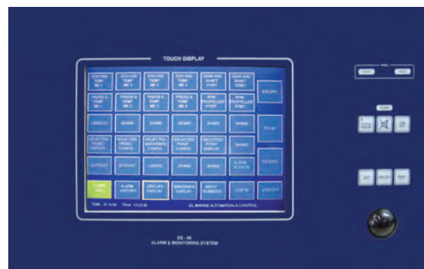
*O.C..P-( OPERATOR CONTROL PANEL)
